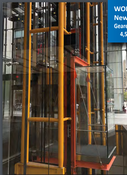
APPLE STORE Michigan Avenue, Chicago, IL In-Ground Hydraulic Passenger 4,000 lb. Capacity
